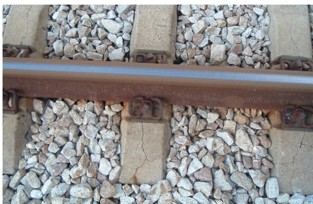
Figure 1. Concrete railway sleepers affected by ASR.
